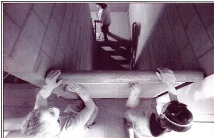
SENIORS RYAN DALLOWAY , left, and Shelby Powell-Hicks sand stairway railings at the Orange County Rescue Mission's Village of Hope on Friday.
